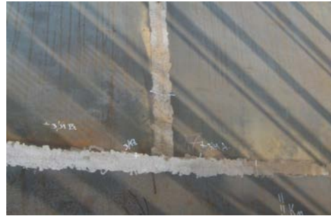
Figure 3. Overshoot of the compounds of the layer to the height of the base material on the inner side of the tank
