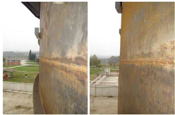
Figure 12. Generating layer of the storage tank in the zones of joints between segments of a shell
