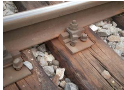
Figure 2: Decay and defects due to rusty water coming from the fastenings
